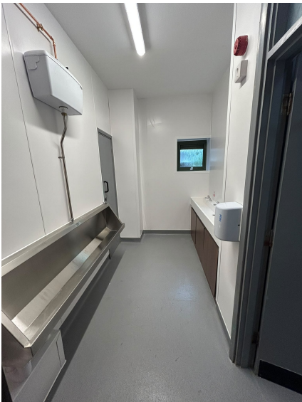
Urinal, cistern and basin run in the boys' WC
